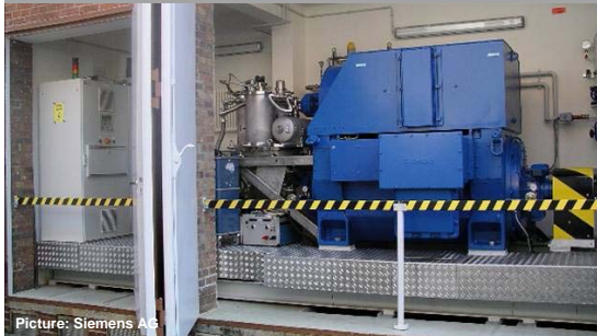
4 MVA Synchronous Generator (1G)
