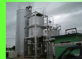
Water treatment system
